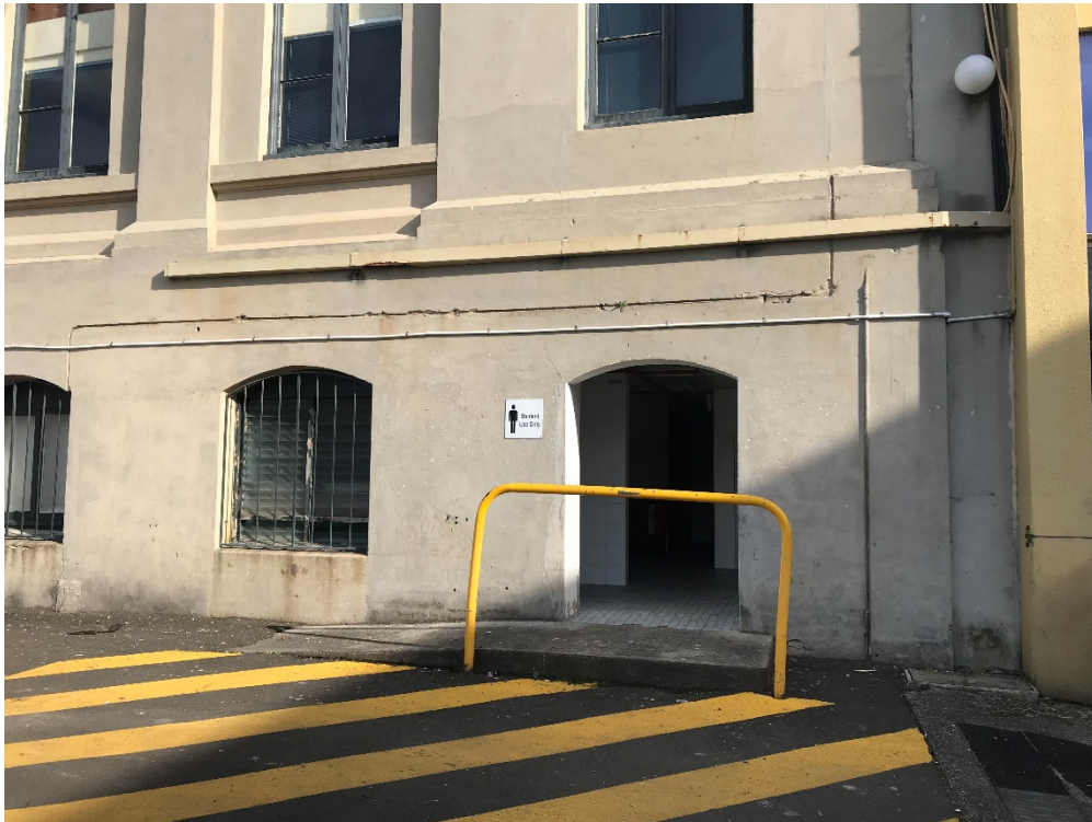
Figure 9: Close up image of the existing openings and ramped entry along the eastern elevation of the Doyle Wing, close to the northeast corner of the building.
