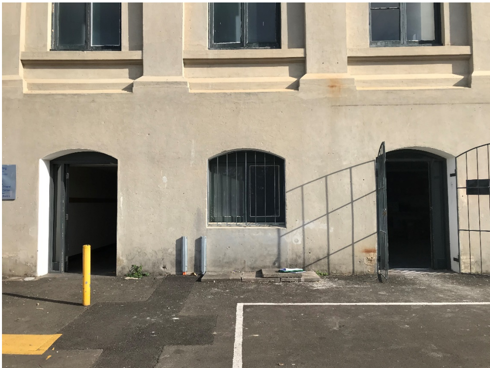
Figure 8: Close up image of the existing openings along the eastern elevation of the Doyle Wing. The window joinery and security grilles are later additions.
