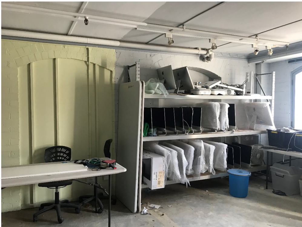
Figure 10: Internal image of a storeroom within the area to be refurbished. It is proposed to reopen the arched openings shown infilled here.
