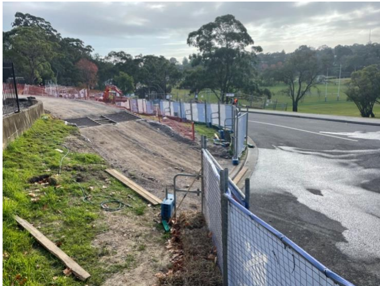
Figure 2 Rumble grid, no visible mud tracking on school roads
