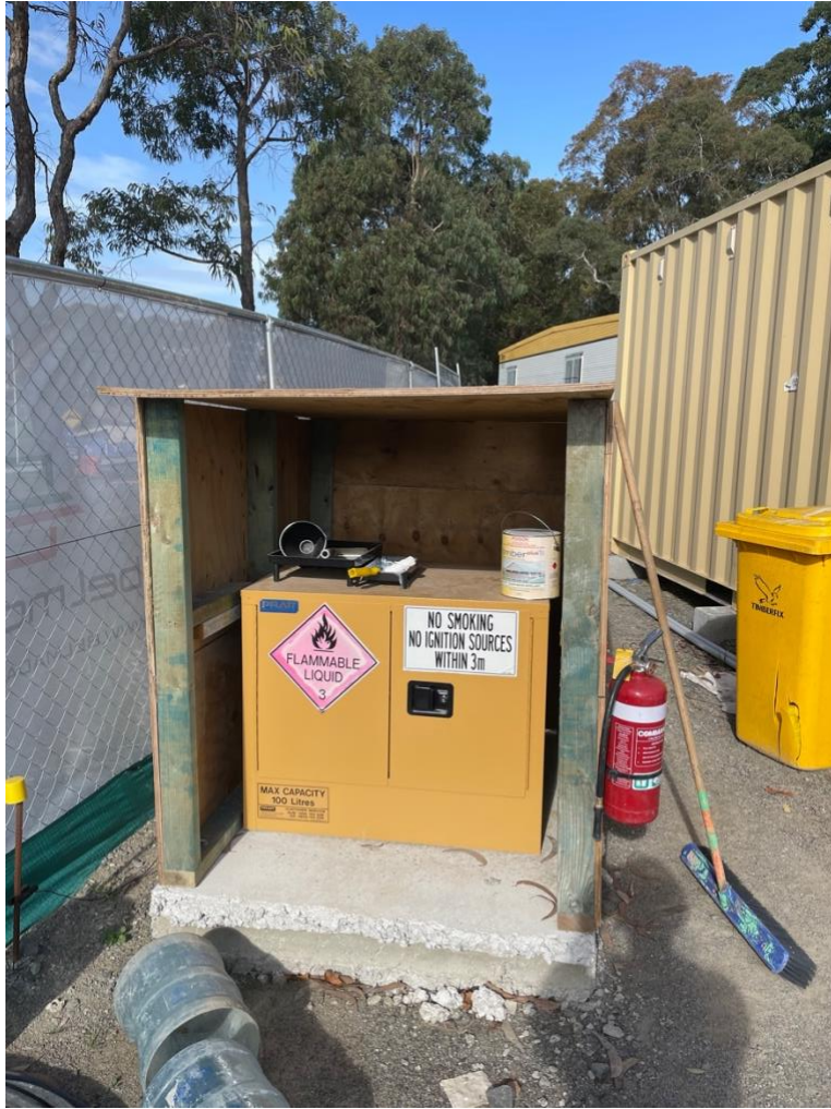
Figure 7 Flammable liquid storage cabinet
